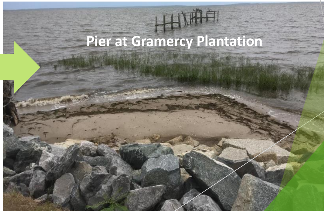
After Hurricane Michael
